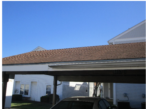
Shingle lift at the carport
