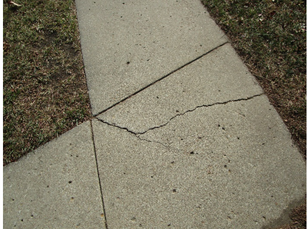
Common sidewalk cracks
