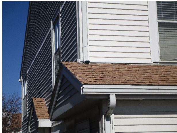
Downspout drainage directly onto the roof
