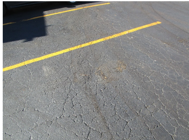
Pavement alligator cracks
