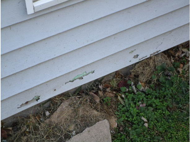
Siding damage at Building 5859
