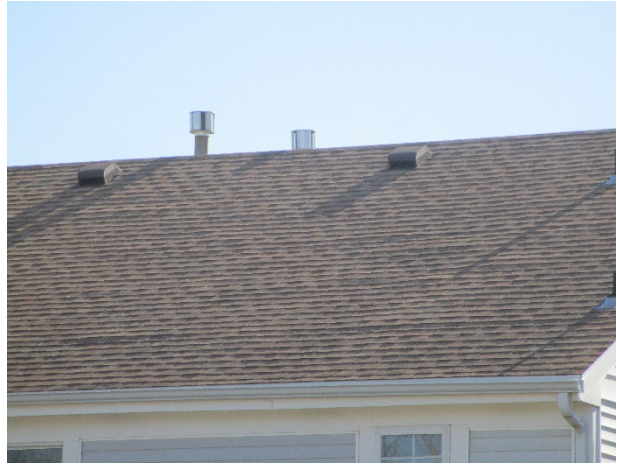
Shingle lift at Building 5803
