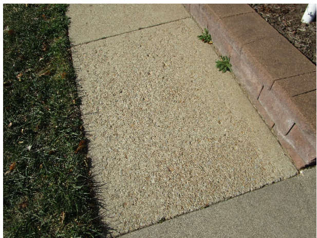
Common sidewalk concrete spall
