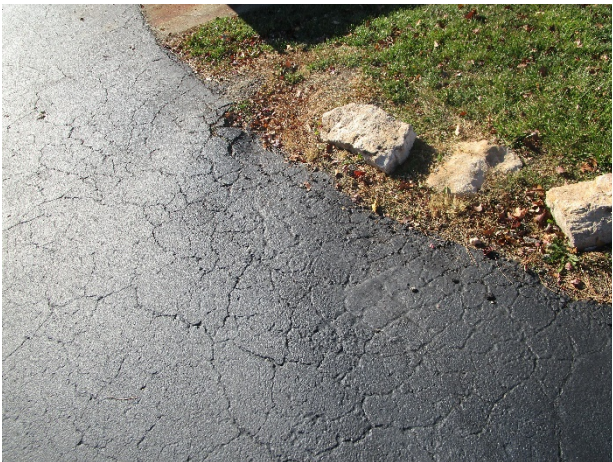
Pavement alligator cracks
