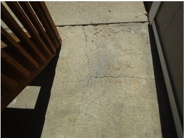
Sidewalk cracks at Building 5817
