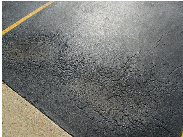
Pavement cracks and settlement
