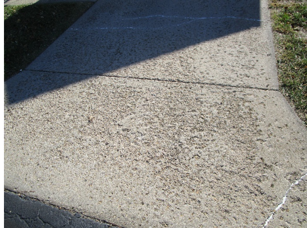
Concrete spall at Building 5831
