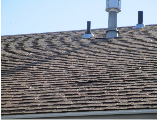
Shingle lift at Building 5821
