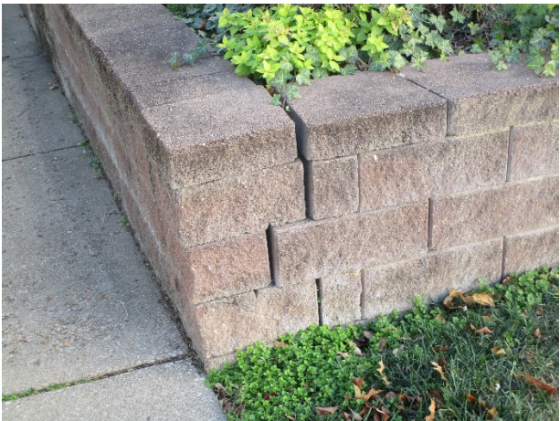
Retaining wall settlement
