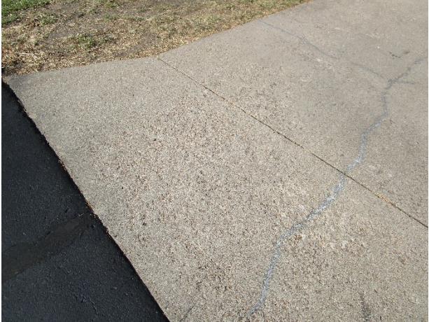
Driveway cracks and concrete spall at Building 5843
