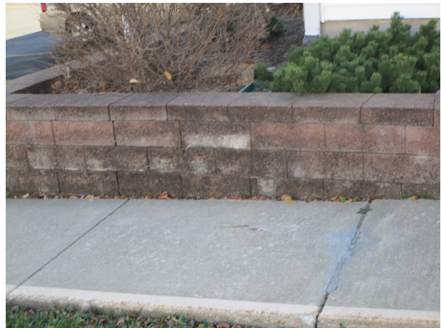
Retaining wall efflorescence
