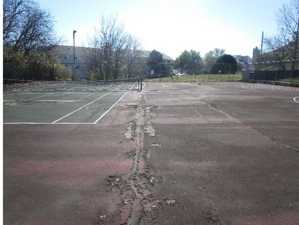
Sport courts overview; Note cracks and coating deterioration
