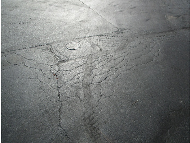
Pavement alligator cracks
