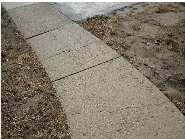
Common sidewalk cracks and concrete spall
