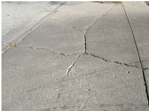
Concrete apron cracks
