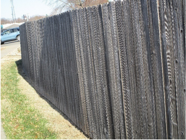
Leaning fence section
