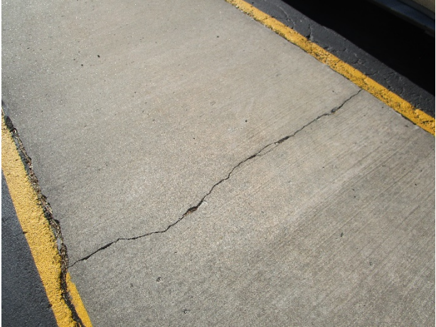
Common sidewalk cracks
