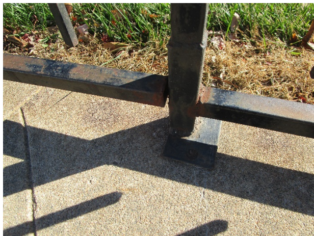
Rust and fence damage
