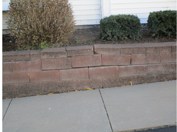
Retaining wall settlement
