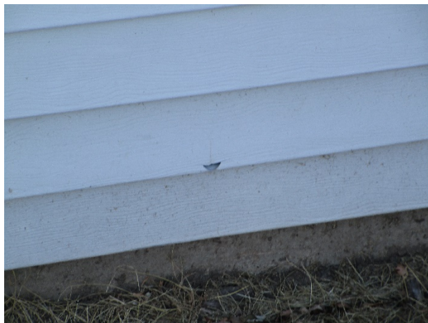
Siding damage at Building 5849
