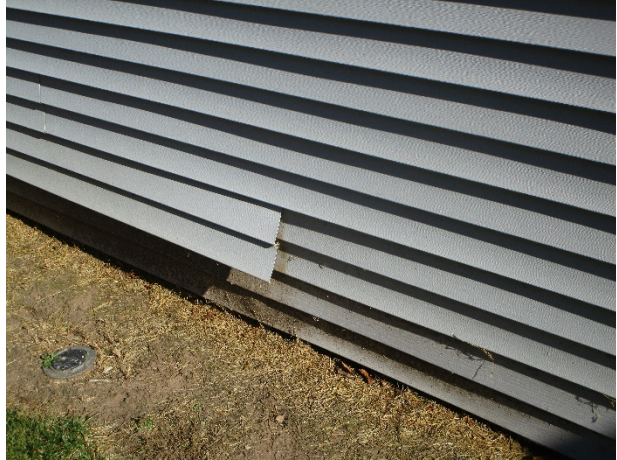
Loose siding at 5835
