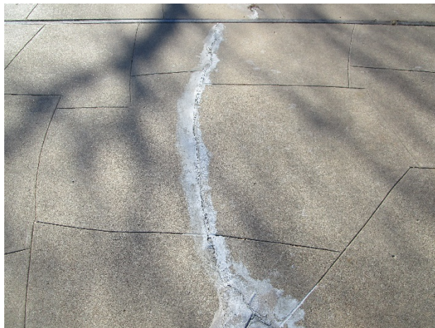
Pool deck cracks
