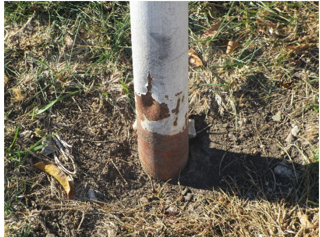
Rust at the base of the light pole
