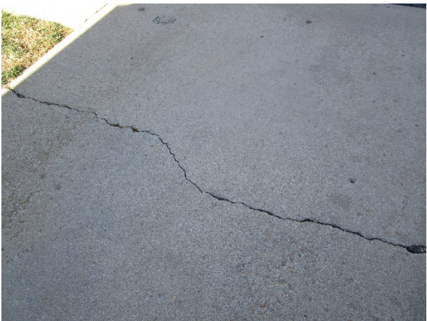
Driveway cracks at Building 5821
