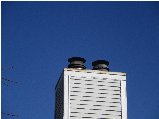
Metal chimney cap; Note rust
