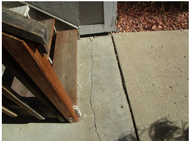
Sidewalk cracks at Building 5829
