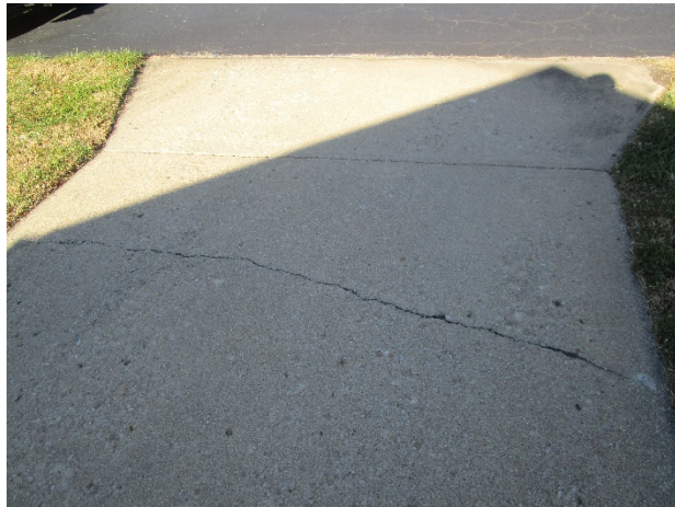
Driveway cracks at Building 5837
